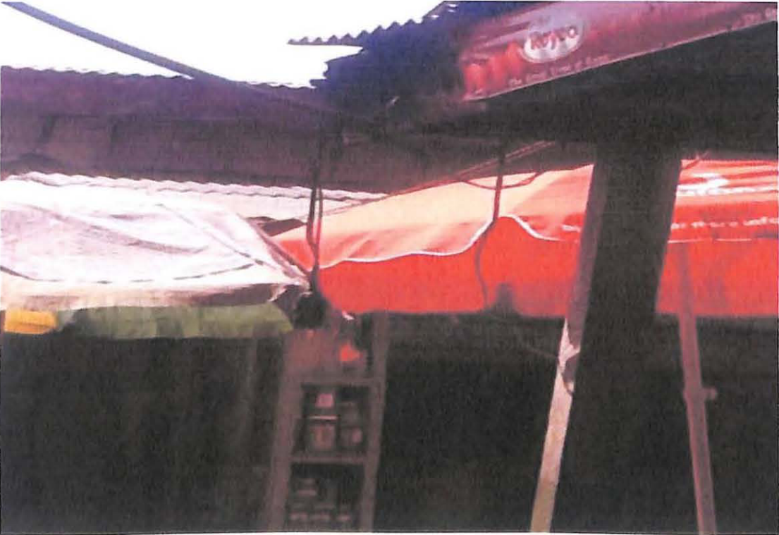
Figure 4: Scenes of suspected Illegal electrical connection
