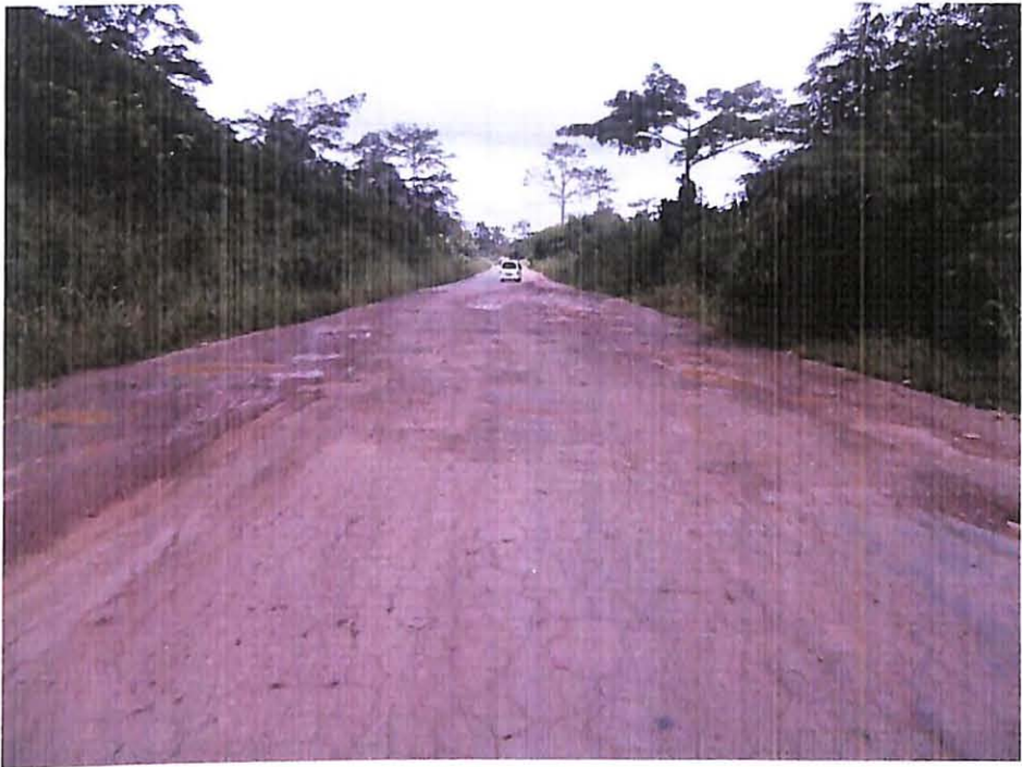
Figure 6: Cracks caused by freight overload. Source, GHA
