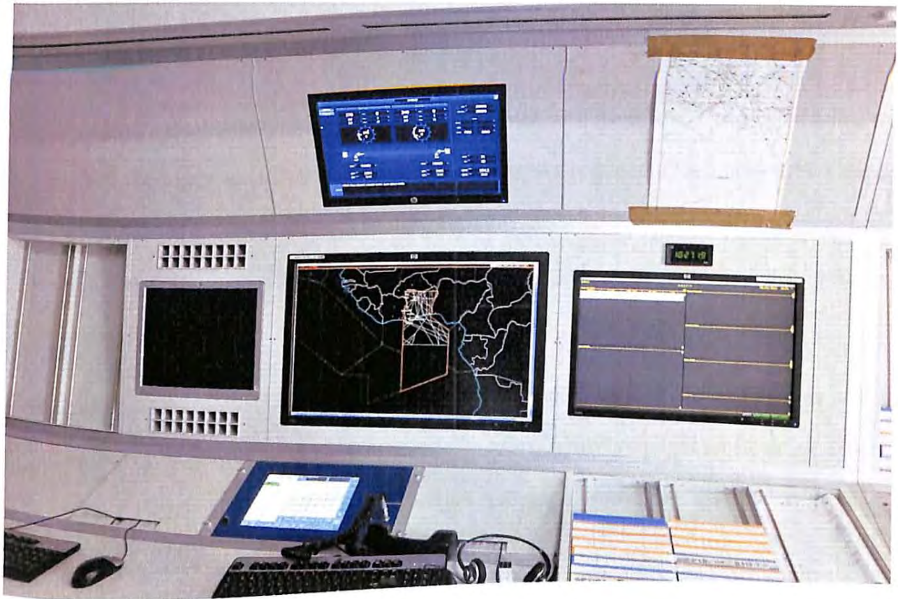
Figure 10: Automatic Dependent Surveillance-Contract/Controller Pilot Data Link Communication (ADSC-CPDLC) installed in 2012
