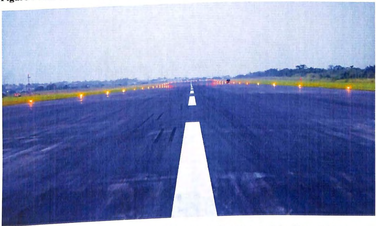
Figure 8: Hi-Tech Aeronautical Ground Lighting (AGL) System at the Kumasi Airport
